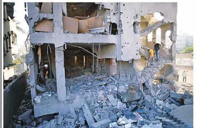
People inspect a destroyed building in the Nuseirat refugee camp in central Gaza, on July 17, 2024.
