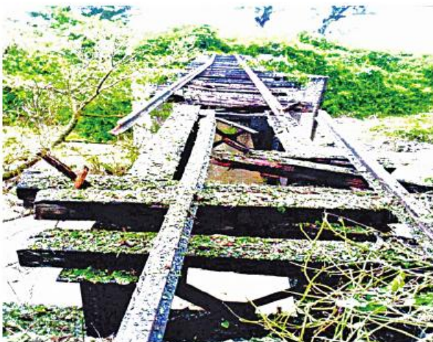
Photo shows the damage caused to the 80-foot long Yaybaukgyi railway bridge by KIA mine attack.
