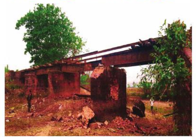
Photo shows the KIA-destroyed section of the 20-foot long Tawet railroad bridge.
