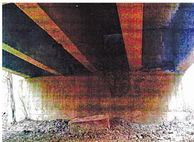
Photo shows the KIA-destroyed section of the 50-foot long Tawet creek motor road bridge.
