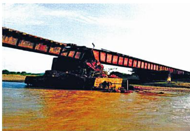
Photo shows the damage caused to the 320-foot long Nankhwin creek railway bridge.
