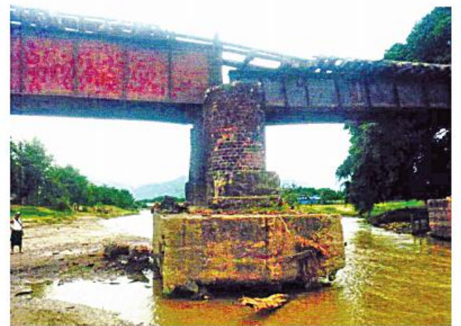
Photo shows the 320-foot long Nankhwin creek railway bridge mined by KIA.
