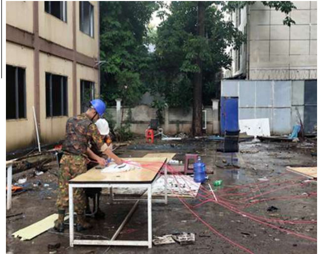
Preparing to demolish the illegal 7-story residential building used for online fraud and gambling operations in Shwe Kokko, Myawaddy District, Kayin State, using explosives.
