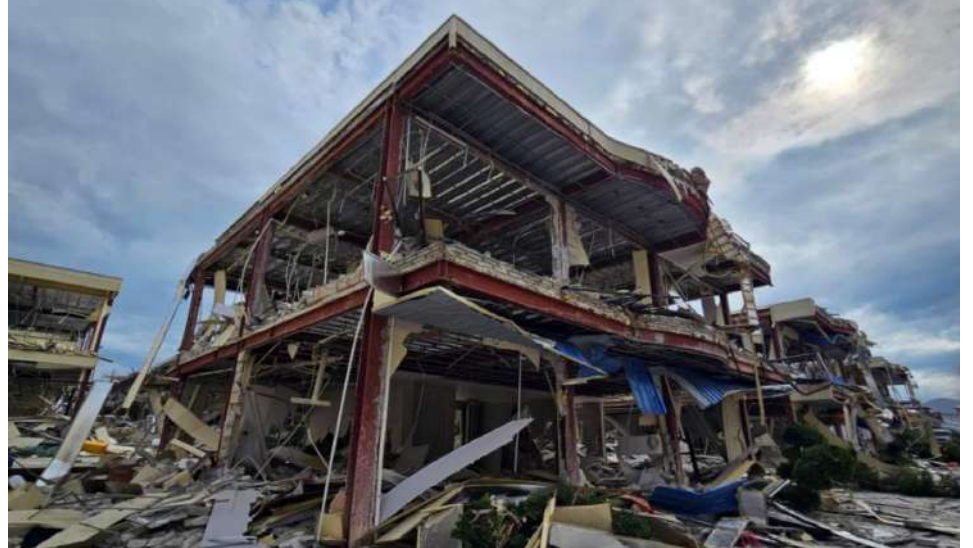
Scenes of buildings being demolished and destroyed; these structures were used for conducting online scam gambling operations within the KK Park area.
