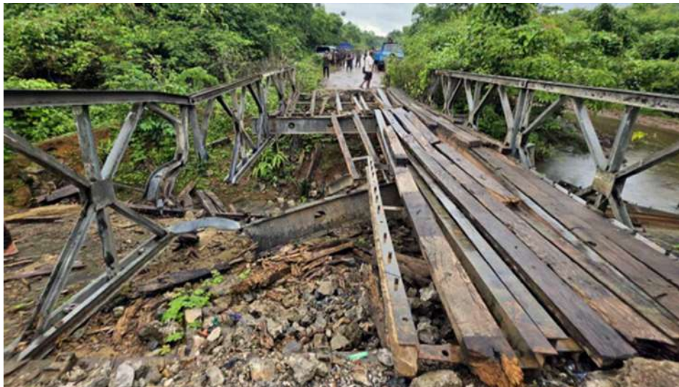
Damage to the Mile-40 Bridge caused by terrorist insurgents' explosive attacks.
